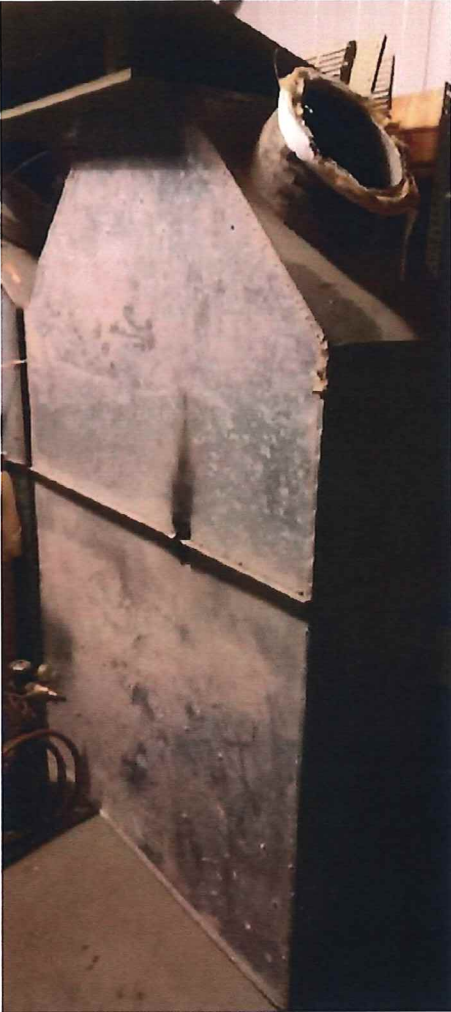
Figure 4: Courthouse Mixing Box
