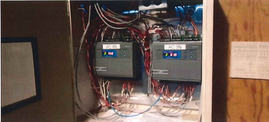
Figure 7: Courthouse Air handling Unit Controls
