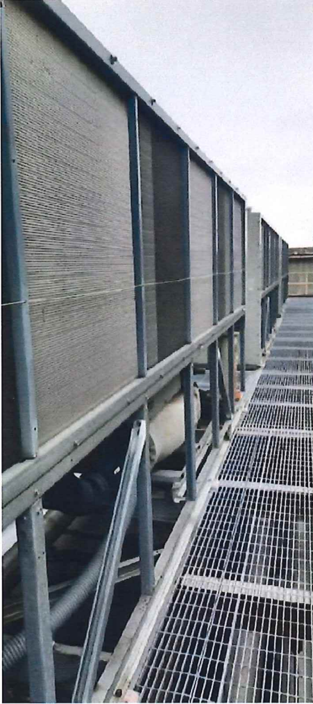
Figure 5: Courthouse Air-Cooled Chillers
