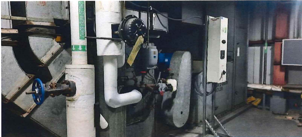
Figure 1: Courthouse Hot Deck/Cold Deck Air Handling Unit
