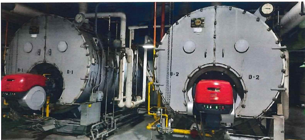
Figure 3: Courthouse Steam Boilers
