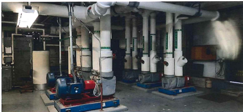
Figure 2: Courthouse Chilled Water Pumps
